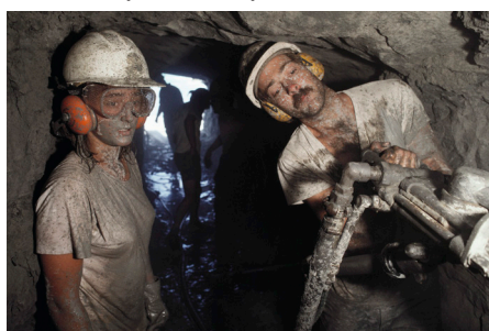
Fig. 8. John Wilson and Corrie Williams. Drillers! Here, these two long term volunteers are drilling a series of holes for explosives in a tunnel at Dinosaur Cove. Corrie's job was to hold the drill steady when John began each hole so the tip remained in the same spot on the irregular rock face. Neither of them had done anything like this previously. One of the many examples of participants learning new skills on the job for the project to succeed. (Photograph by ©Peter Menzel/ menzelphoto.com .)
