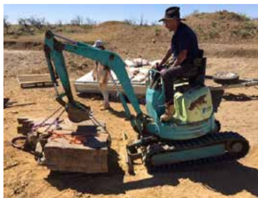
Dave, you're going to need a bigger digger to lift that trackway slab!
