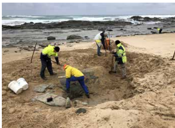
Nick van Klaveren, Alan Tait, John Wilkins and Corrie Williams digging out the hole in warm hats and waterproof jackets
