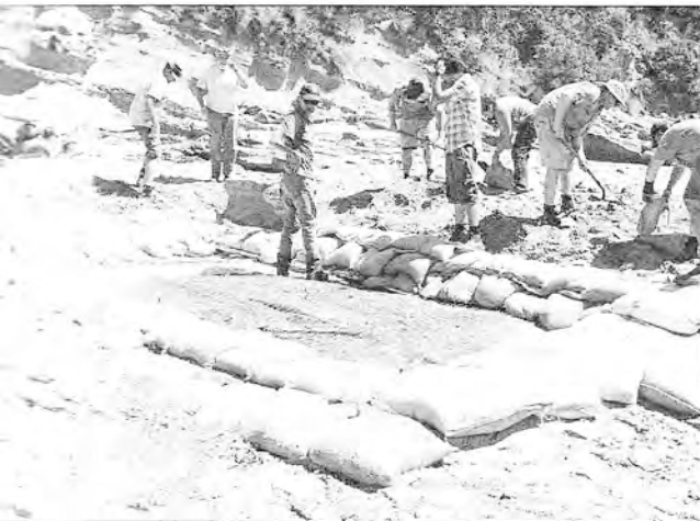
The system before the storm - how the finished system looked before "the Storm of the Century" damaged it.
