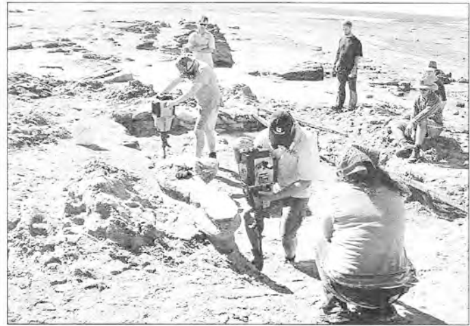
At the start of the dig, drilling holes around the perimeter of the excavation for the rock bolts.
