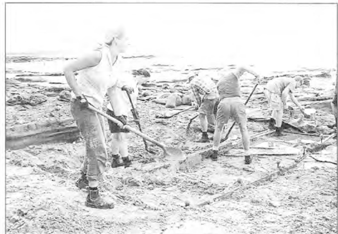
Removing the sand that accumulated on top of the system during high tide.
